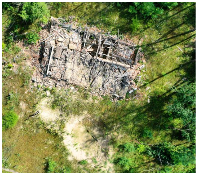
Aerial view taken by a drone showcasing a damaged building during non-technical survey (July 2023).
